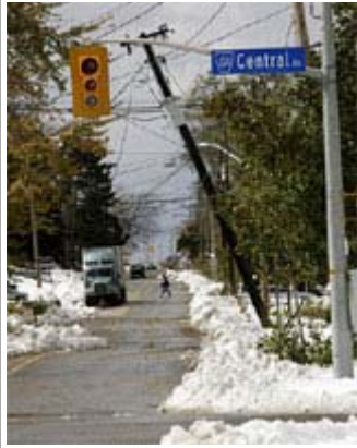
Damaged power poles are seen in the city of Fort Erie, Ont., after a snow storm ripped through felling trees and damaging homes. The Canadian Niagara Power Company estimates it could take up to five days to completely restore service. (CP / Nathan Denette)
