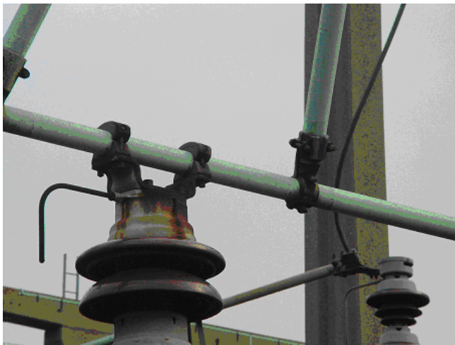
Figure 12: Busbar Clamp Corrosion
