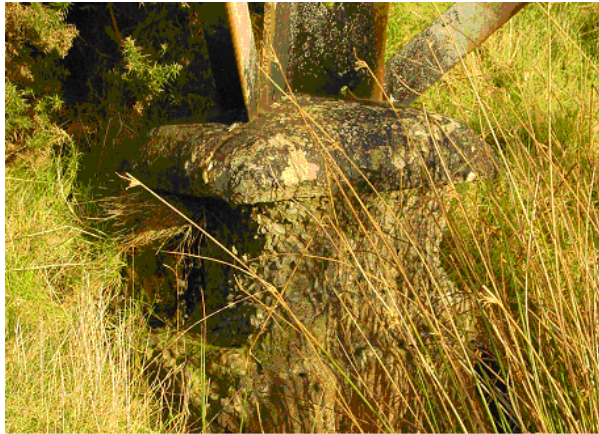
Figure 7: Deterioration of Overhead Line Steel Tower Foundations
