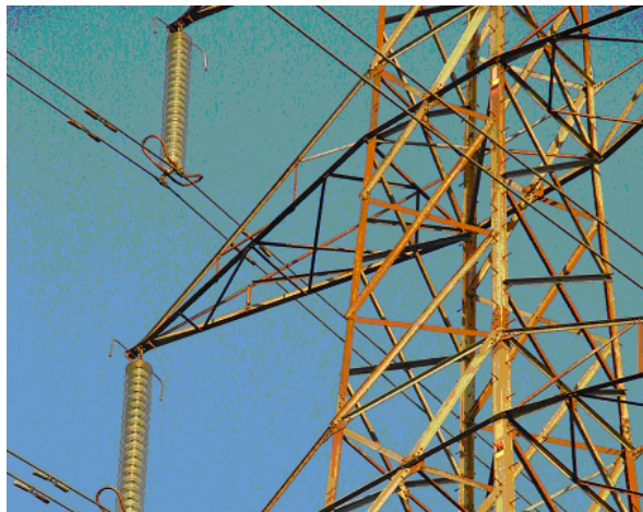
Figure 6: Lattice Overhead Line Steel Tower Corrosion
