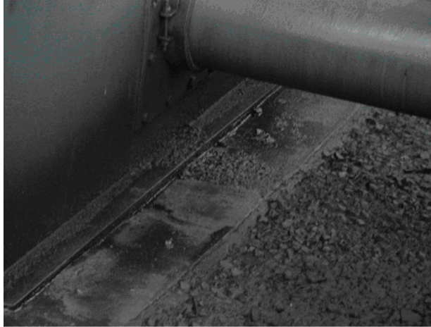
Figure 13: Transformer Insulating Oil Leakage
